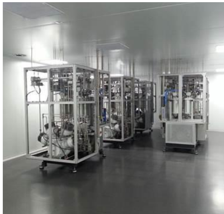
ASPI's Carbon-14 enrichment facility
